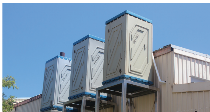
Three BioGill bioreactors replaced the ageing Dissolved Air Flotation (DAF) system.
