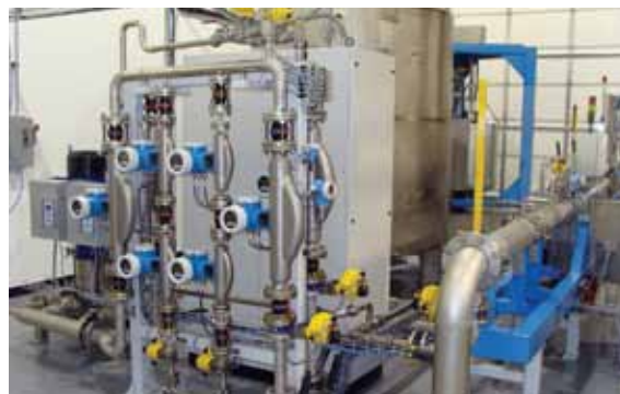
Figure 3. At a certified flow calibration rig, flowmeters are calibrated to meet applicable standards, such as Endress+Hauser's ISO/IEC 17025 A2LA Accredited Calibration Laboratory in LaPorte, TX.
